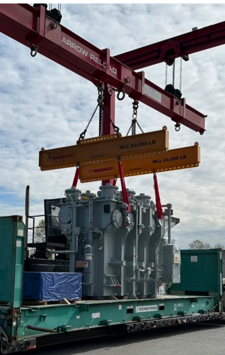
Transformer, approx. 57,000lbs.
